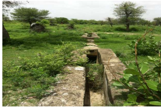
Figure 6: Drains Built in Agore Area of Johad of Anant Ramji of Ramgarh-Shekhawati
